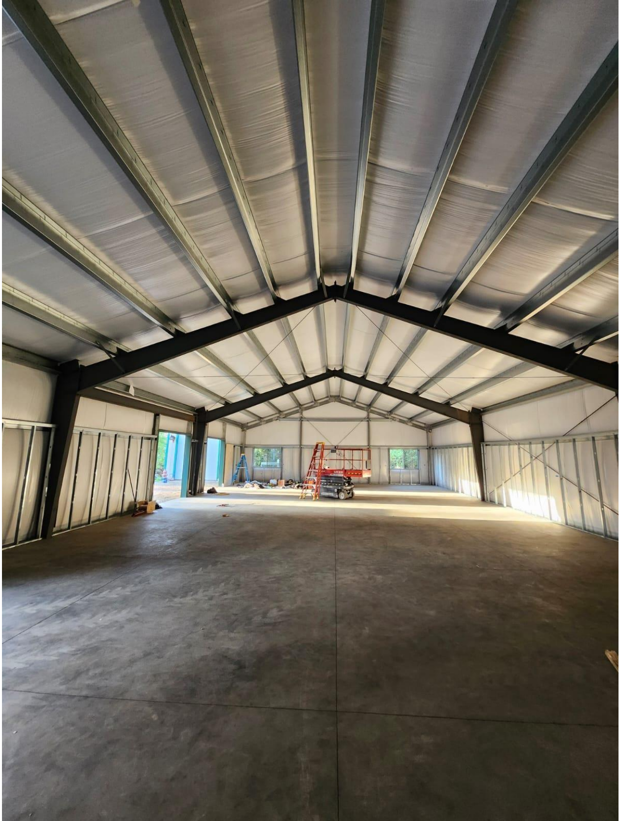
PHOTO OF FINISHED WORK. FRANCHESKA'S STORAGE INSTALLATIONS LLC.
