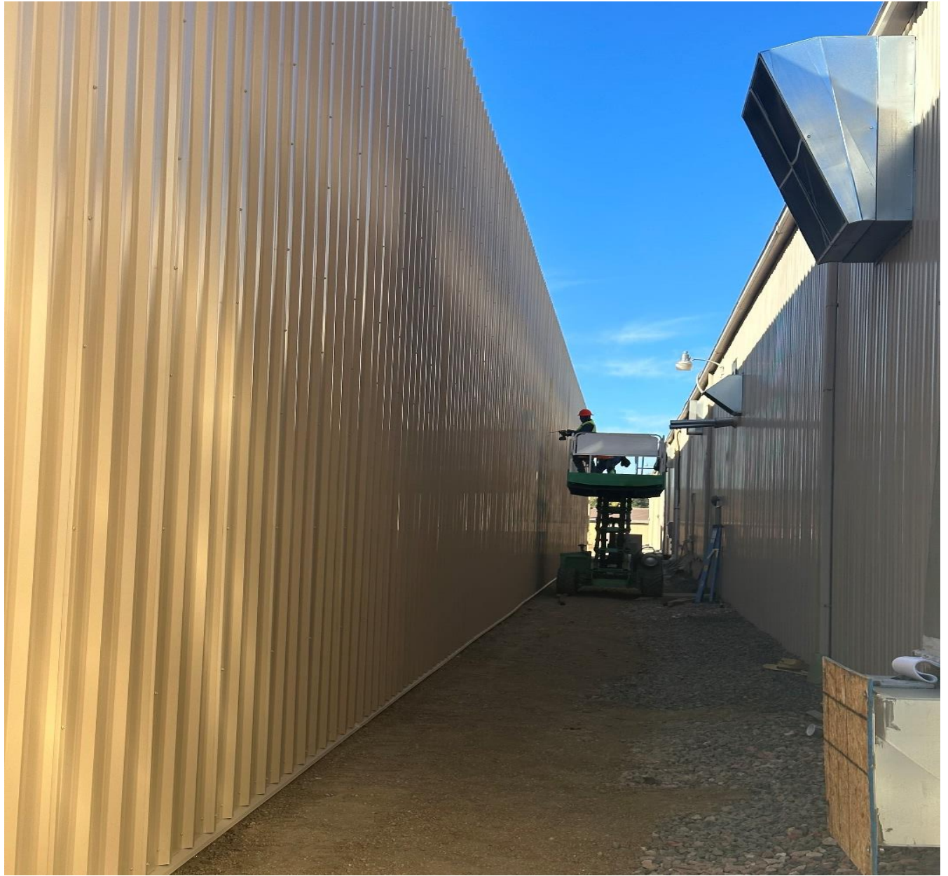
PHOTO OF FINISHED WORK. FRANCHESKA'S STORAGE INSTALLATIONS LLC.
