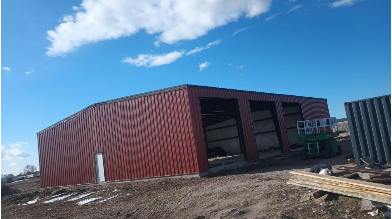
PHOTO OF FINISHED WORK. FRANCHESKA'S STORAGE INSTALLATIONS LLC.
