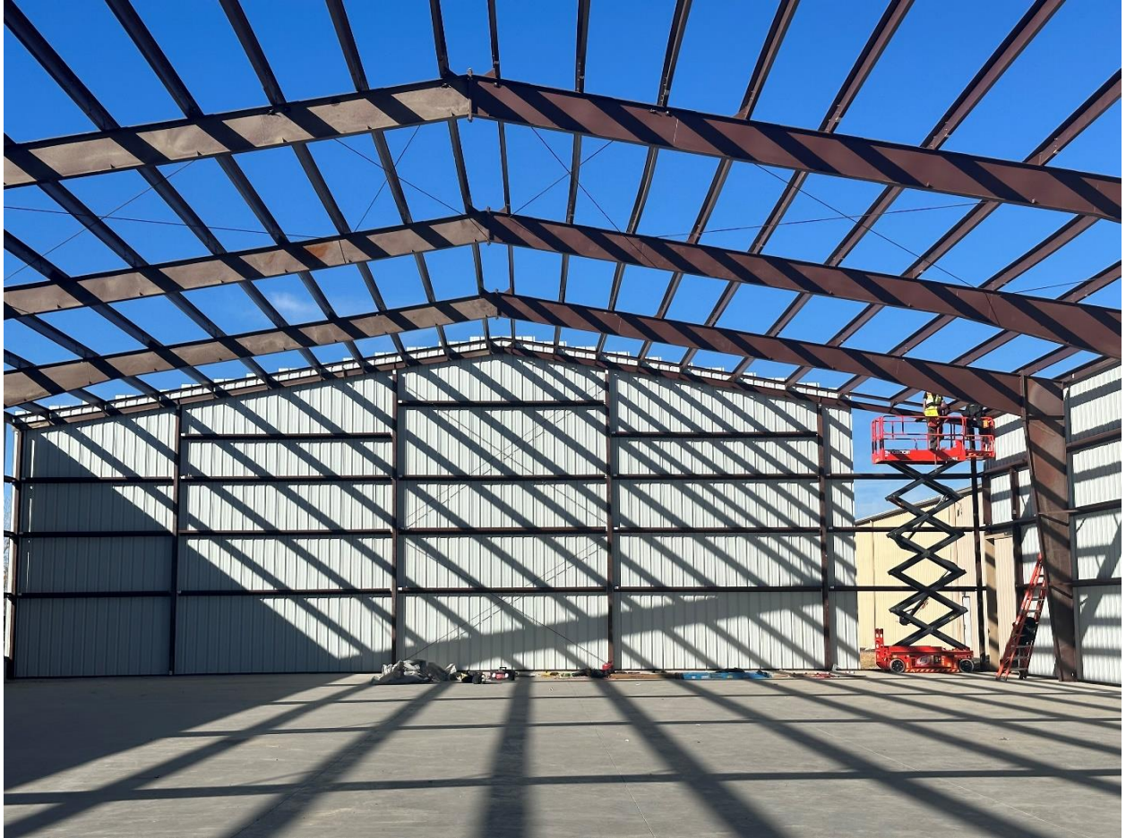
PHOTO OF FINISHED WORK. FRANCHESKA'S STORAGE INSTALLATIONS LLC.
