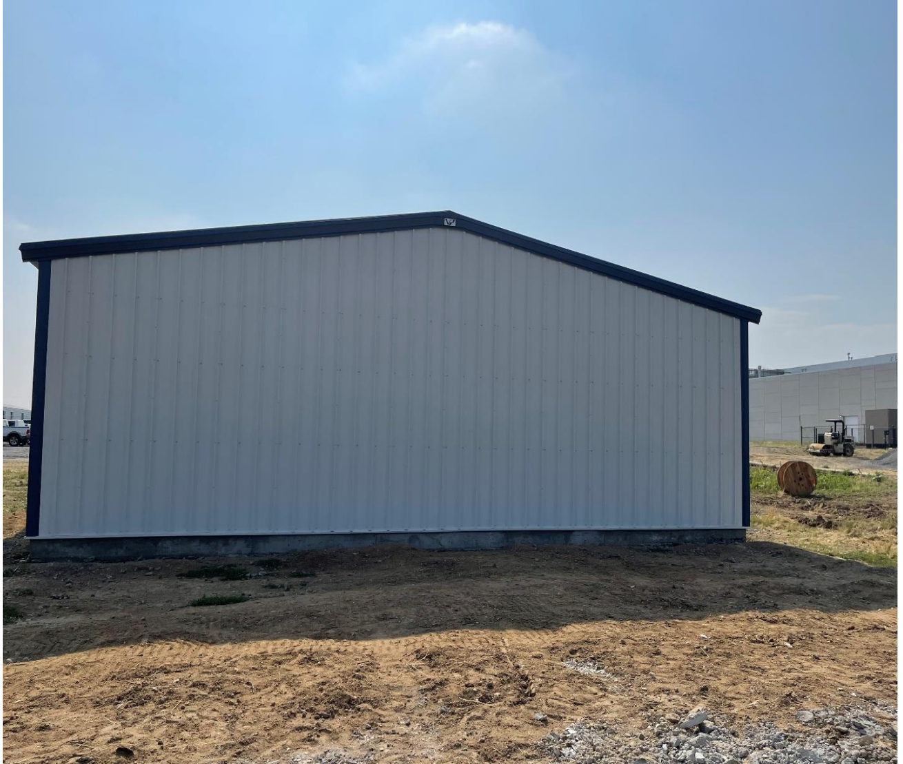
PHOTO OF FINISHED WORK. FRANCHESKA'S STORAGE INSTALLATIONS LLC.
